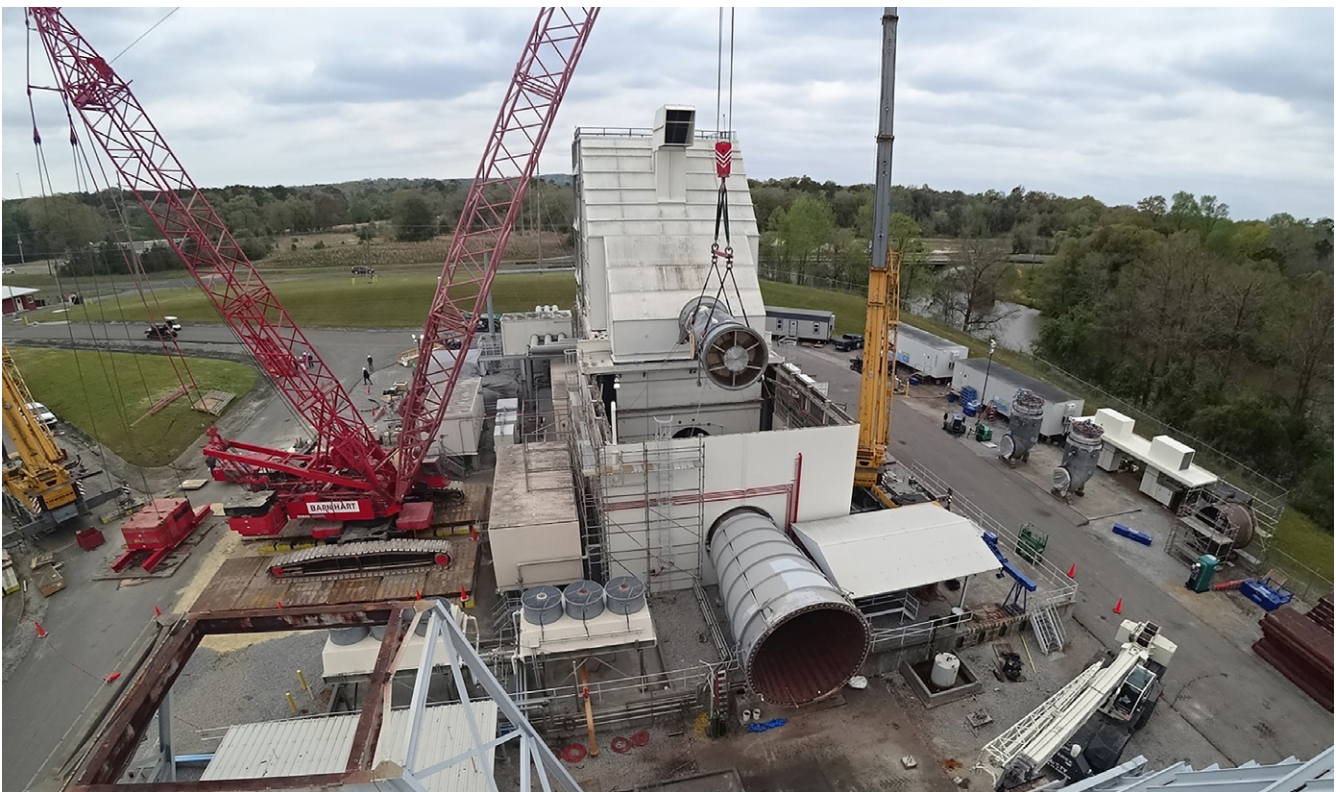
An old gas turbine is being replaced at a power plant in Convington County, Alabama. It enables the power plant to produce 114 megawatts (MW) of cleaner energy, up from an average of 102 MW.
