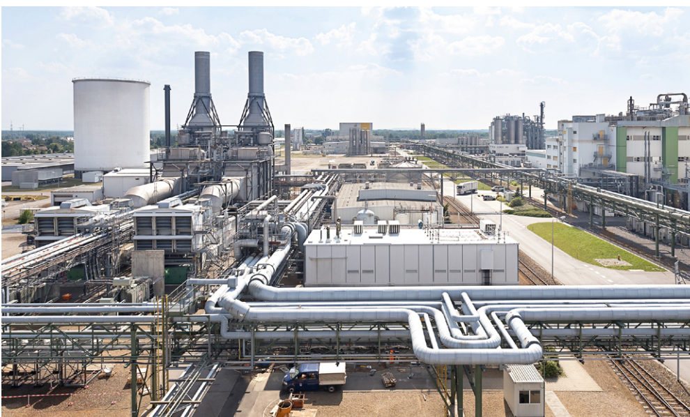
Modernizing an industrial power plant: At the BASF Schwarzheide industrial plant a new efficient gas turbine was installed, as well as a battery storage system for black-start capability.
