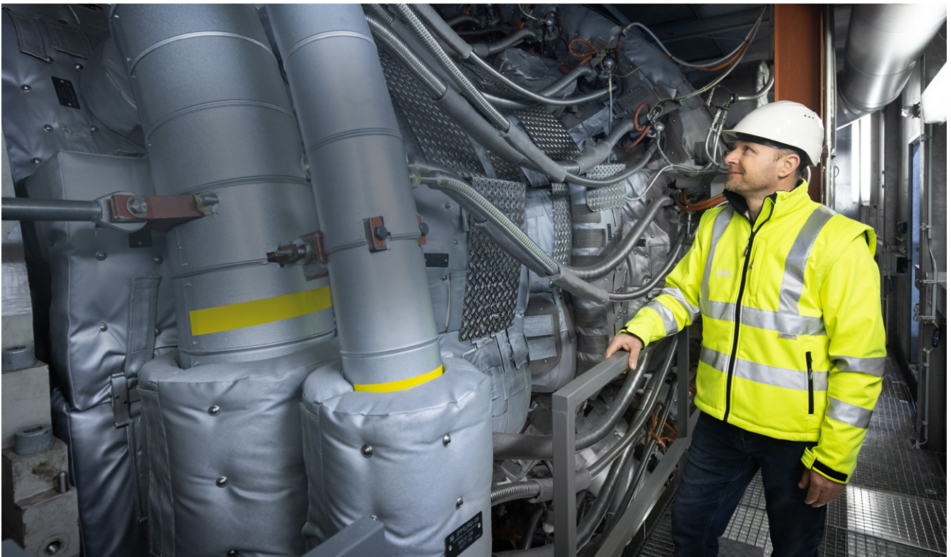
The thermal power plant in Theiss, Austria, is the first to install a hydrogen-capable gas turbine.
