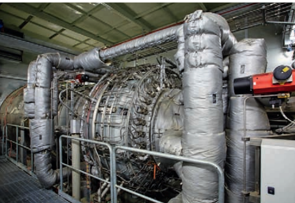
The SGT-800 gas turbine is the centerpiece of the power plant, ensuring highest efficiency and lower emissions.
