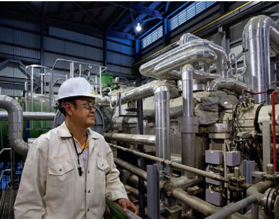
Engineer Cherdchai Yiwlek supervised the construction of the plant. His prime concern: fuel efficiency.
