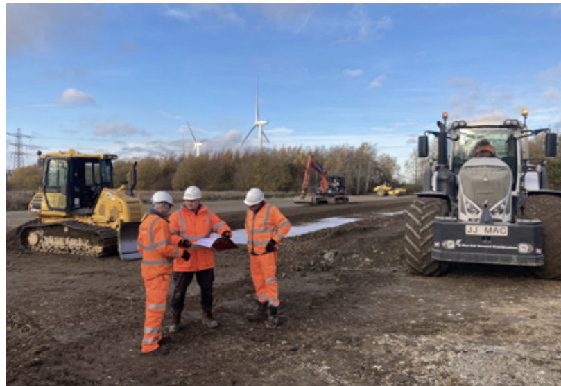
The stone used at the onshore Triton Knoll substation will be transported to the adjacent National Grid Viking Link interconnector project
