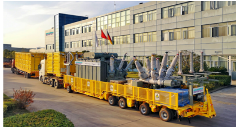
In Zhengzhou: the green mobile substation equipped with a Sensformer™ filled with natural ester oil ready for operation
