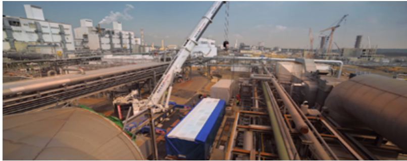
After modernization, the combined cycle power plant at BASF Schwarzheide in Germany is now 10% more efficient
