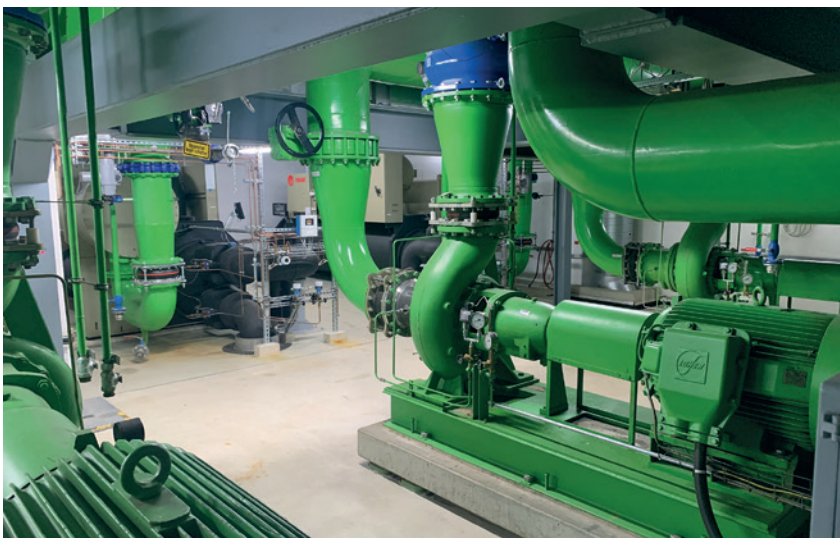
Figure 2. Vattenfall's cooling plant at the heart of the German capital
