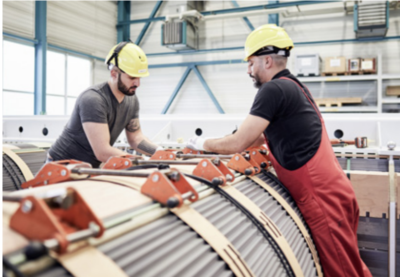
Siemens Energy transformer factory in Nuremberg.
