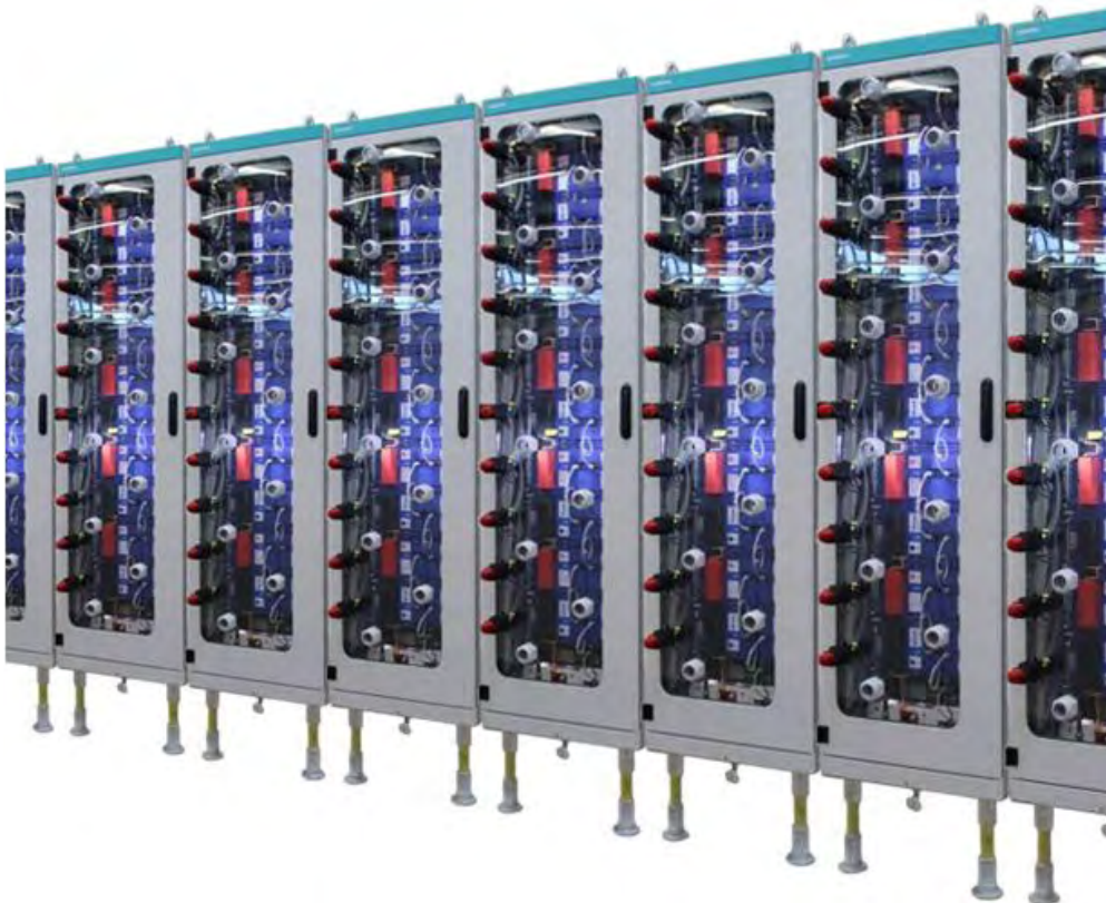
Fig. 5: Supercapacitors actively contribute to stabilizing the grid in times of sudden disturbances.
