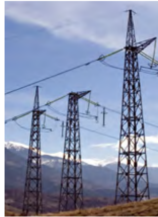
400 kV line in Bulgaria NGLA solution realized with 3EL2
