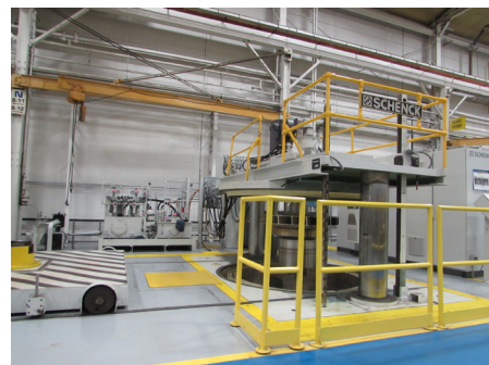
Figure 2: The overspeed test pit. The mandrel assembly is positioned on the cart (far left), which is rolled under the overspeed machine where it is fastened to the spindle. It is lowered into the pit, and a vacuum pump evacuates the chamber to minimize the power required to drive the impeller and heat generation associated with windage.
