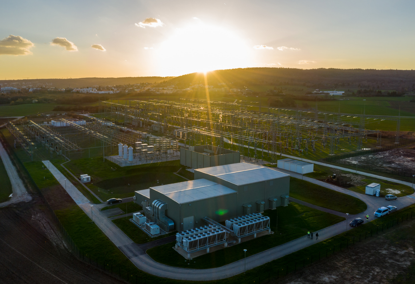
Amprion's STATCOM substation in Kriefel to support the power supply for the greater Frankfurt area in Germany with its almost six million inhabitants.
