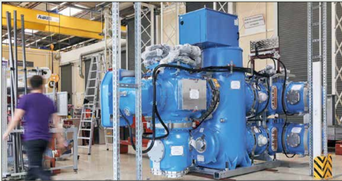
F-gas-free switchgear at the Siemens Energy switchgear factory in Berlin
