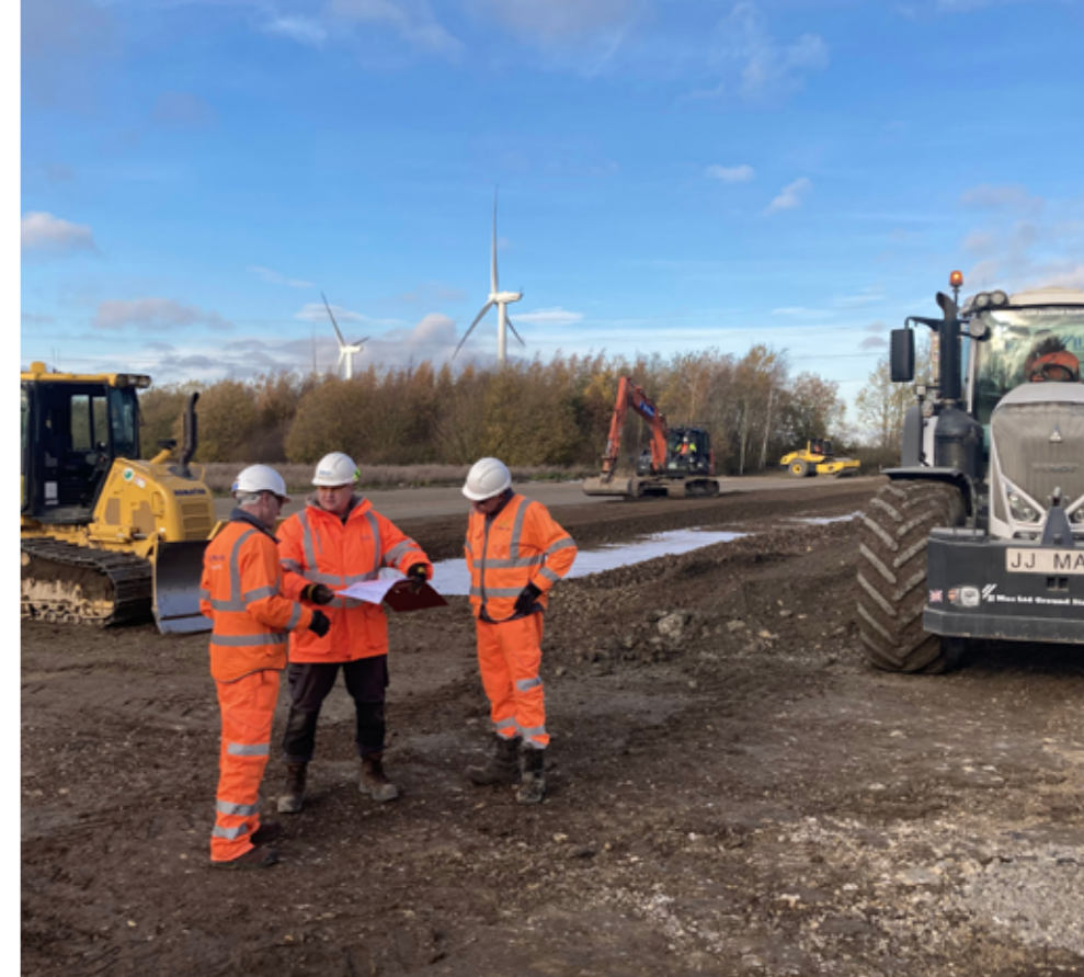
The stone used at the onshore Triton Knoll substation will be transported to the adjacent National Grid Viking Link interconnector project
