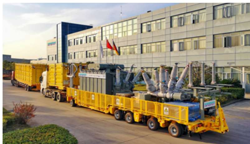
In Zhengzhou: the green mobile substation equipped with a Sensformer™ filled with natural ester oil ready for operation
