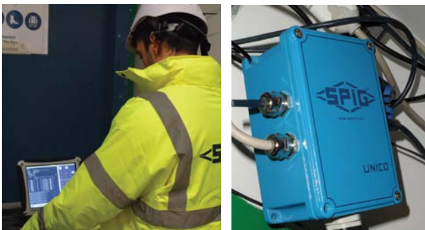
UNICO installation on an air-cooled condenser
