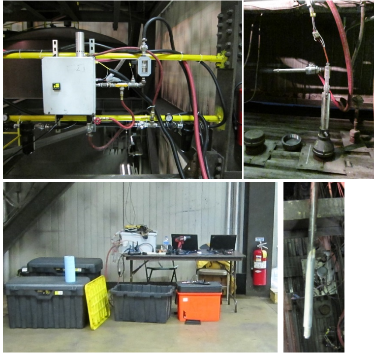
Figure 2. Corrosion monitoring system (clockwise from upper left), a) instrument box, b) inserted probe, c) corrosion probe with sensor elements, d) control computer.
