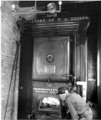
B&W Boiler, Thomas Edison’s Laboratory
